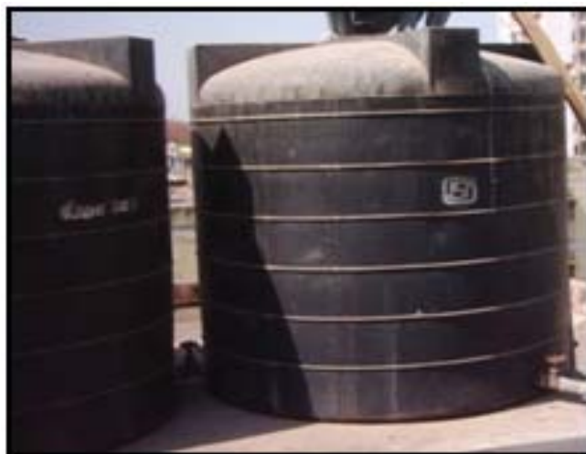
Open Overhead Tanks
